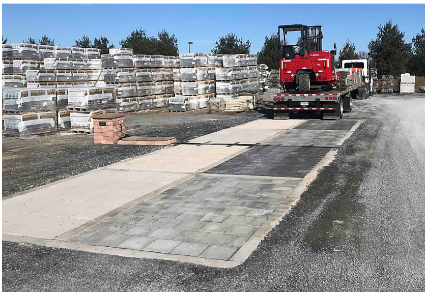
Test pad with slabs and planks on concrete and aggregate bases subject to tractor-trailer loads.
