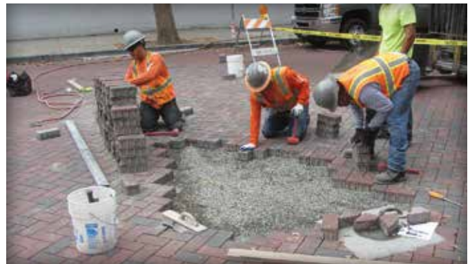
Figure 3. Once smoothed and joined with undisturbed materials at the opening perimeter, the bedding receives concrete pavers.
