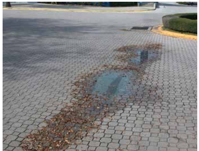
Figure 18. Depressions are caused by settlement of the base or subgrade and are easily spotted by the puddles formed after rain events.
