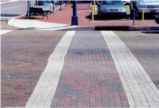
Figure 23. Horizontal Creep is easily spotted in ICP areas that were constructed straight, but over time develop a wave in the pattern.
