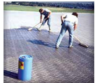
Figure 10. Urethane is applied with squeegees to stabilize joint sand between pavers on aircraft pavement.
