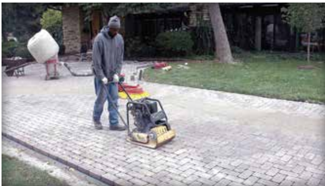
Figure 19. Edge restraint is spiked into the dense-graded base berms so it can hold the pavers in place during compaction and service.
