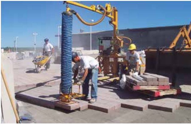
Figure 12. Self-contained vacuum lifter with boom
