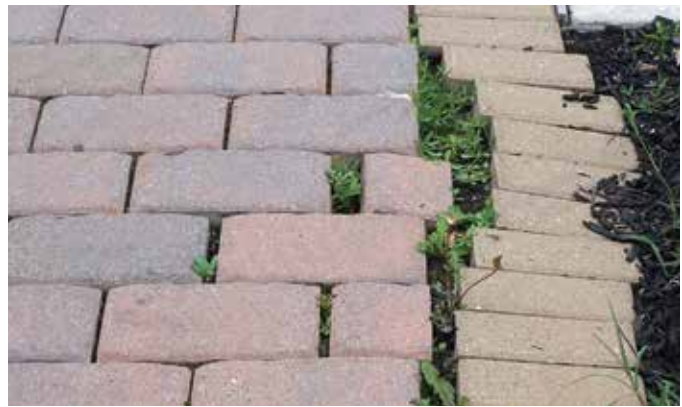
Figure 19. Lack of an effective edge restraint has allowed the pavers to separate and compromise the structural capacity of the ICP.
