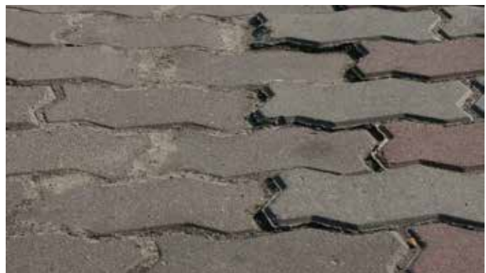
Figure 21. Faulting can be seen as a line of pavers being lifted above the neighboring units.
