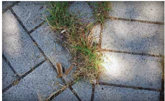
Figure 9. Weeds indicate sediment accumulation and lack of surface cleaning to remove it.
