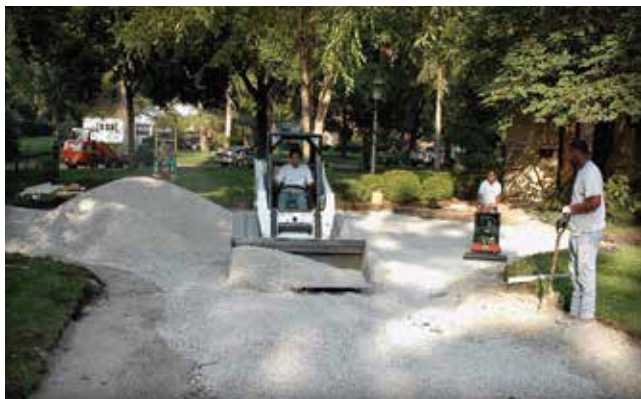
Figure 17. Perimeter berms made with dense-graded base are in place prior to placing open-graded aggregate in the driveway.
