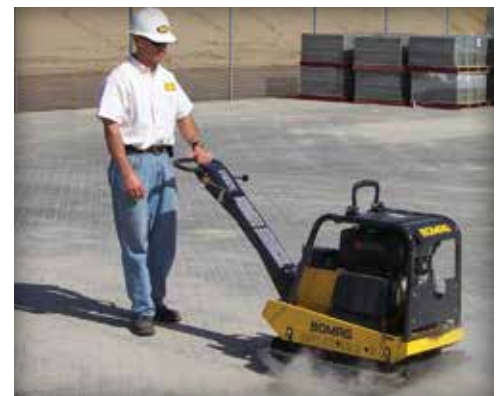
Figure 13. Final compaction should consolidate the sand in the joints of the concrete pavers.
