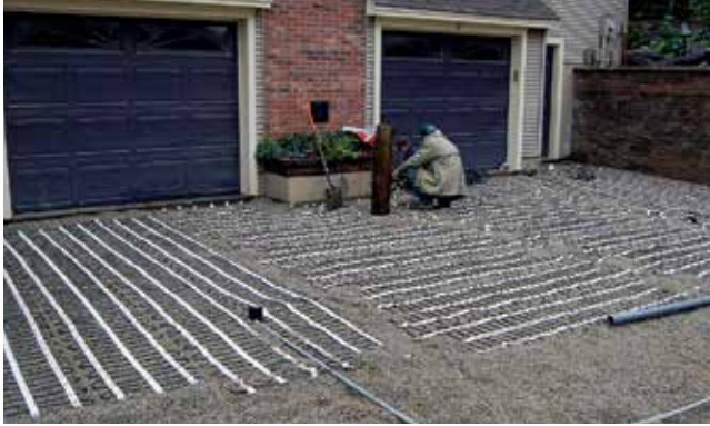
Figure 10. Electric heat tape snow melt system is installed in the bedding layer of permeable interlocking concrete pavement.
