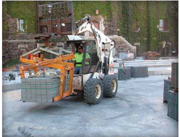
Figure 8. Clamps are an efficient method of moving cubes of pavers around the site, and can eliminate the need for wooden pallets.
